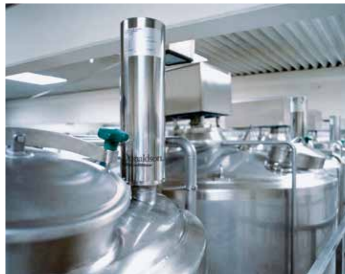
Filter housings for the aeration on storage tanks.
